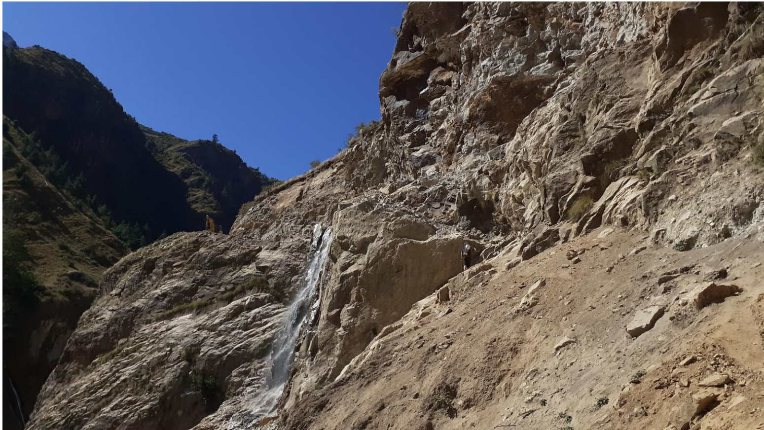
The path/road between Dharapuri and Kermi. Top is in 2017, below is the same section in 2019. It has been destroyed whilst blasting a route for the 'new road' to Simikot. Passing through this section in 2019 was impossible for mules (they took the long way up and around to the village above). It was passable but very dangerous for us! The worst section was protected by a length of nylon cord attached to a partially buried steel rod fixed rope.
