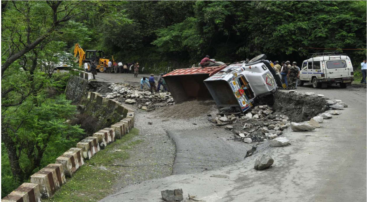
Collapsed road due to the heavy monsoon rainfall. (photo Rachel Antill)
