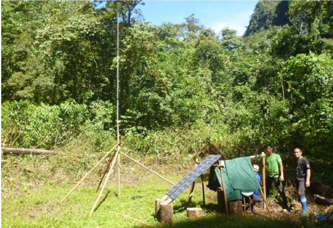
Radio repeater station and solar charger on helipad | Dave Nixon.
