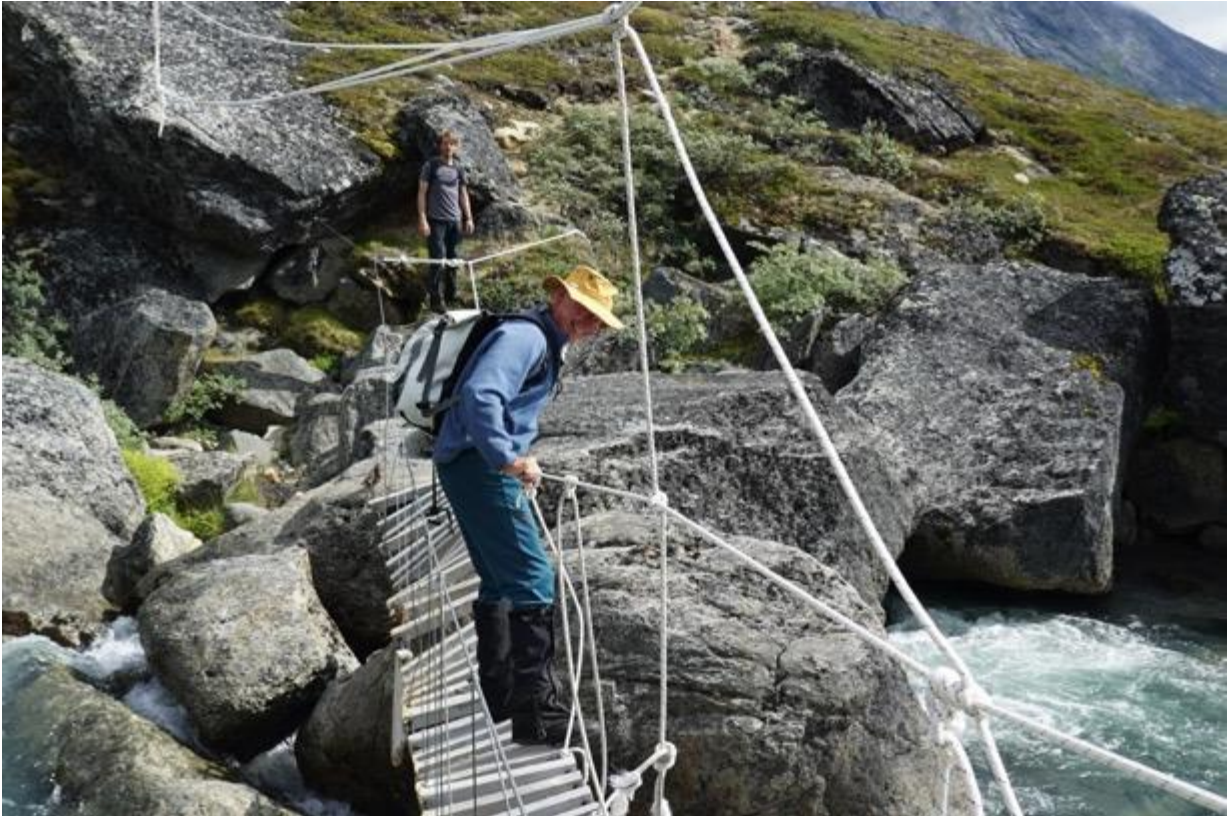
Photo 10: Tim carefully crossing the winter damaged bridge at Point 72
