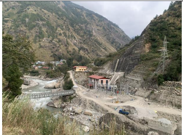
Photo 24. A major development in the Langtang Valley ~20-megawatt hydropower plant already in the final stage of completion which will be connected to the national gridlines.
